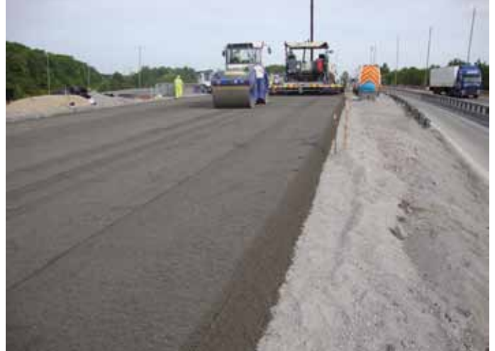
The use of a CBGM subbase and base provided real programme benefits
