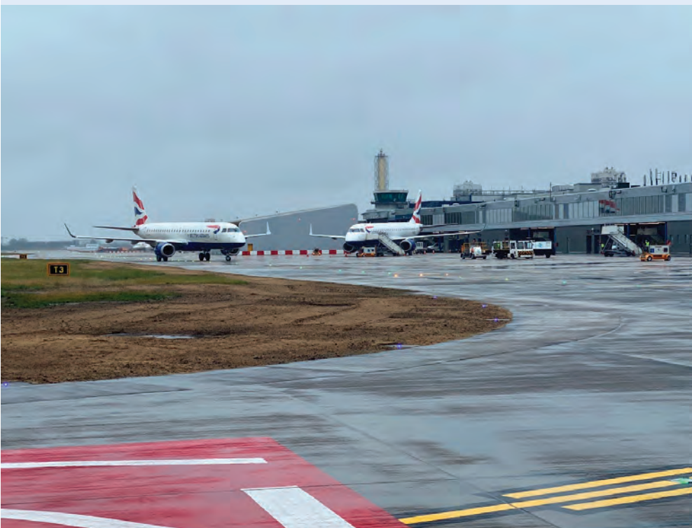
Fjori and Norder collaborated on the recent concrete taxiway reconstruction at London City Airport
